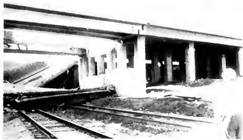
Photo 2. Damaged San Fernando Road overhead [2].
